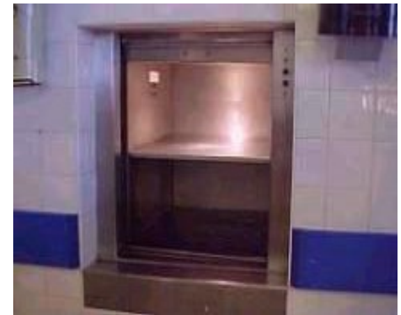
Service Lift Hilton Hotel Cardiff
